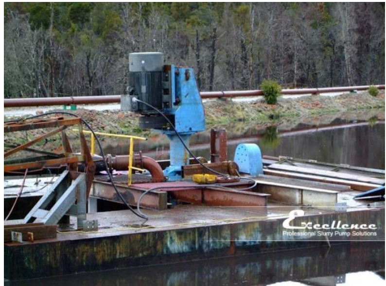
EVHM-6SV in Coal Washery in Australia
